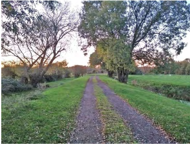
Figure 3: Much of the former rail alignment remains as an elevated embankment suitable for reinstatement (Photo: C. Ross 2019).
